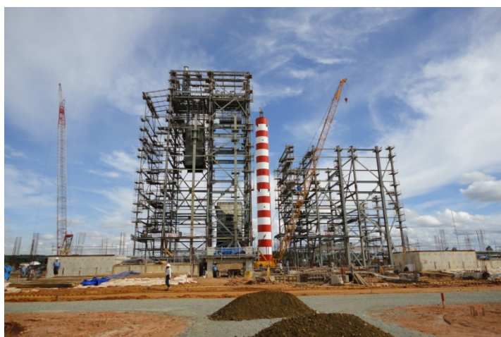
The ground view of 2X30 MW mine-mouth power plant construction site (December 2010)
